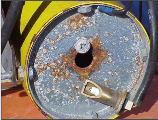
Figure 1. Corrosion of rear cover and electrode. Remove electrode from rear
