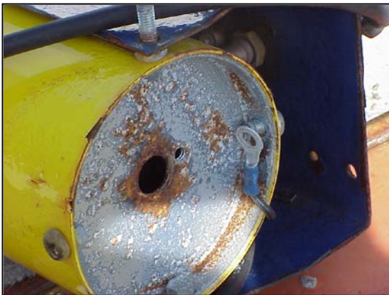
Figure 2. Corrosion of rear cover and ground wire. Remove ground wire from rear cover.
