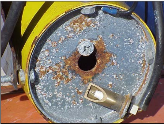
Figure 1. Corrosion of rear cover and electrode. Remove electrode from rear cover.
